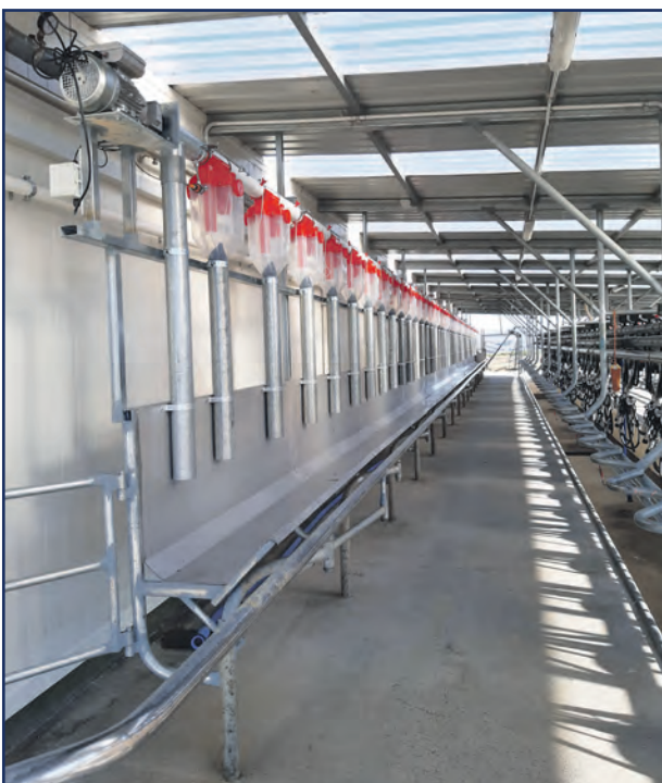
In-shed feed system install, herringbone and rotary.
